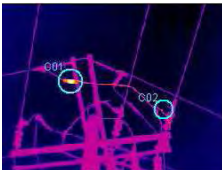
Fig. 5: Bad contact (CO1) on an overhead line connection identified by thermography
