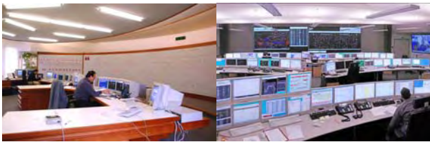
Fig. 18: Former and modern control centre in Carinthia
